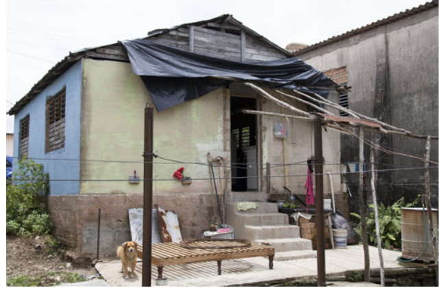
Rear of house showing part of the tin roof missing blowing away during hurricane
